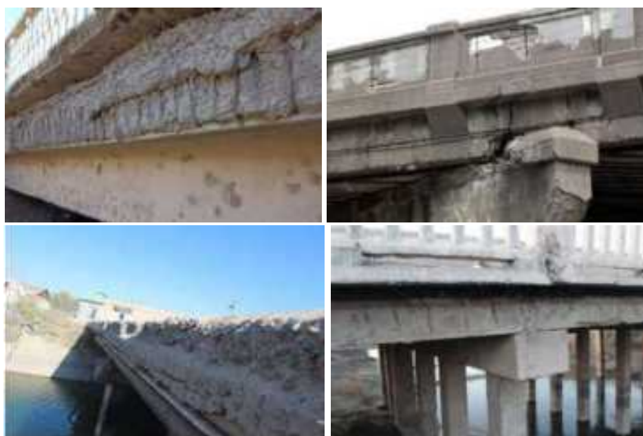
Fig. 2. Damage to the structure caused by malfunctions in the waterproofing system
