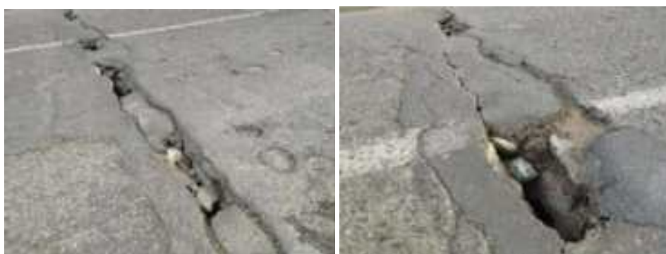
Fig. 3. Defects and damages caused by deformation seams
